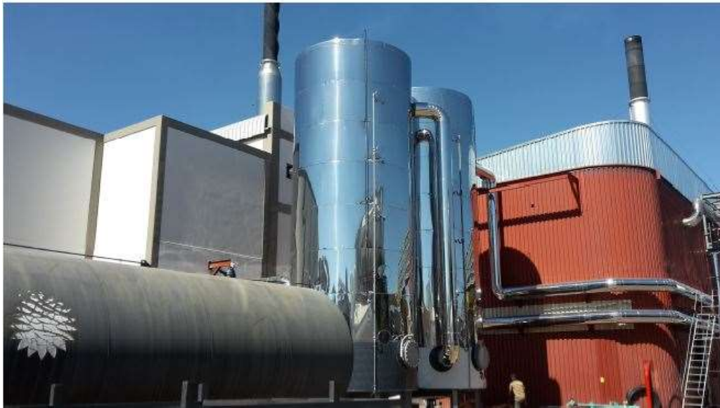
Figure 1.7: EEP thermal biofuel boiler (Namibia EEP - Africa, 2015)
