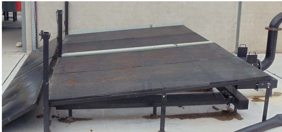
Picture of the drying beds using heat from exhaust.
