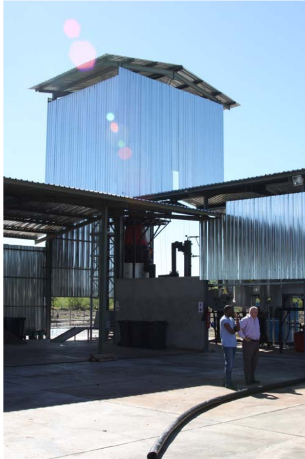
Figure 4.14: The CBEND pilot plant facilities with metal roofs and concrete slabs
