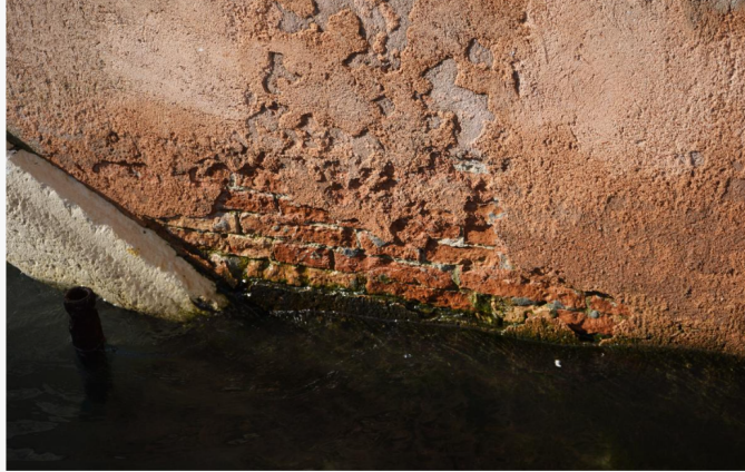
An example of damage done to a canal wall
