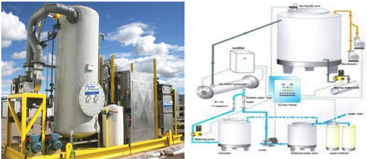
Figure 5.1 Sodium hypochlorite control system (Ampac 2010)
