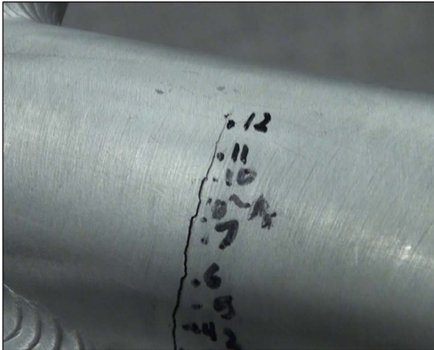
Figure 47: Extent of crack propagation on front side.
