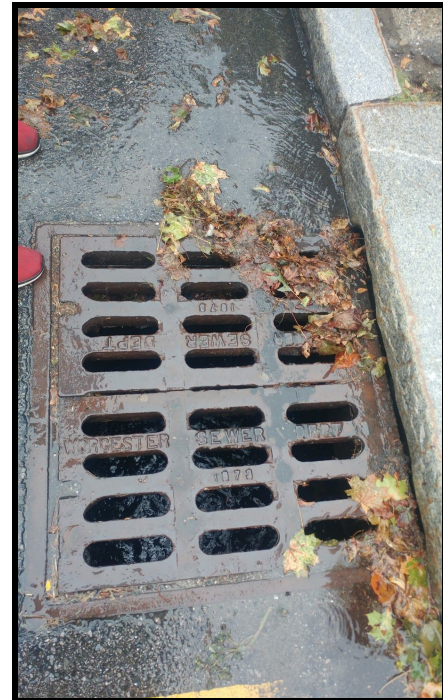
Above: Close up of Institute rd./Boynton St. Drain
