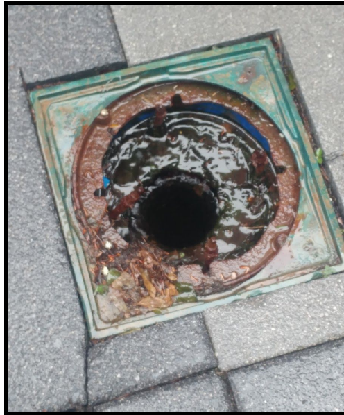
Above: Sidewalk Drain outside Kaven Hall at the bottom of the steps beside Fuller labs
