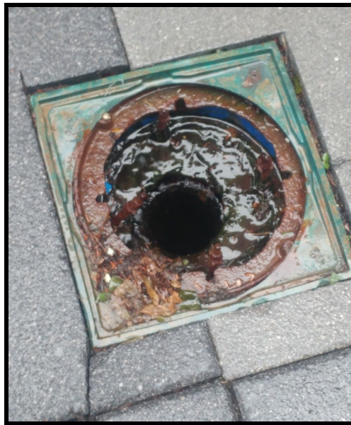
Above: Sidewalk Drain outside Kaven Hall at the bottom of the steps beside Fuller labs
