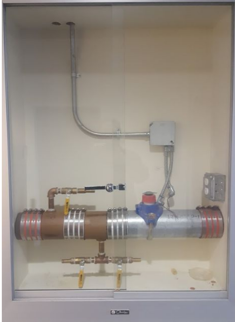
Above: Green roof monitoring site inside East Hall
