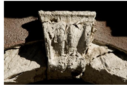
Figure 11: Keystone showing years of deteriorating effects
