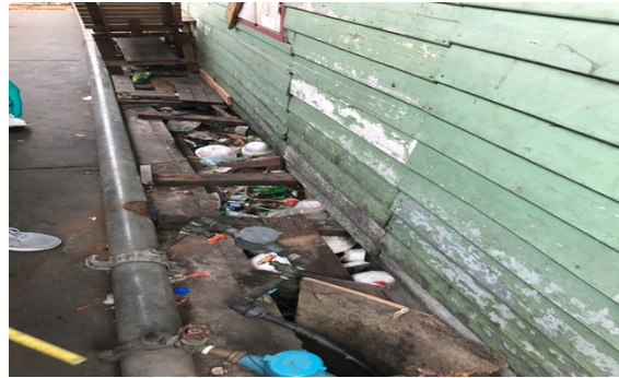
Figure B: Trash Buildup in the Drains Preventing Water Flow
