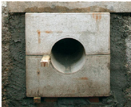
Figure 8: A Gatolo (Sewage disposal, 2012)
