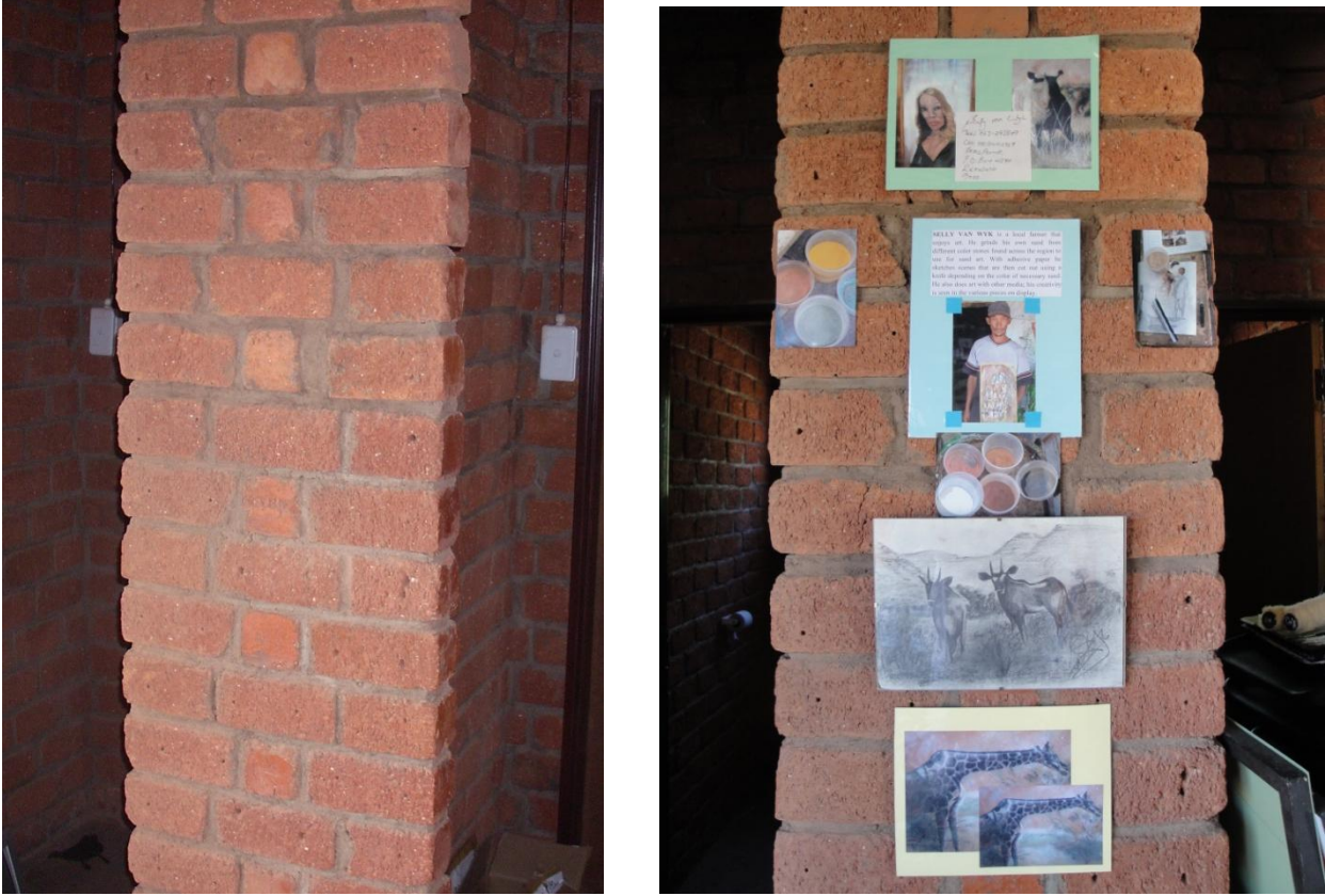
Figure 38: Pillar Before and After
