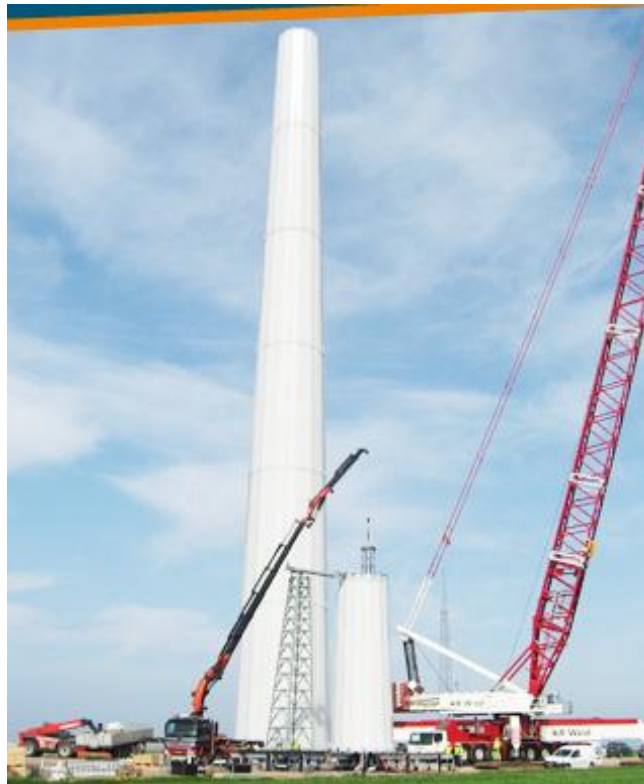
Fig. 4.11 Shell Tower (Andersen Towers, 2011)
