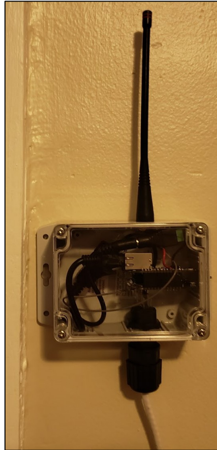
Figure 16. Gateway Mounted on the Wall
