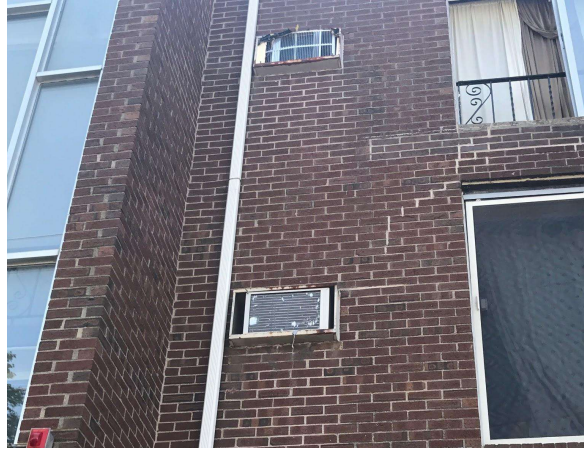
Figure 18: In-wall air conditioners. At this condo on Addison Street the air conditioners were installed in the wall, rather than in windows.
