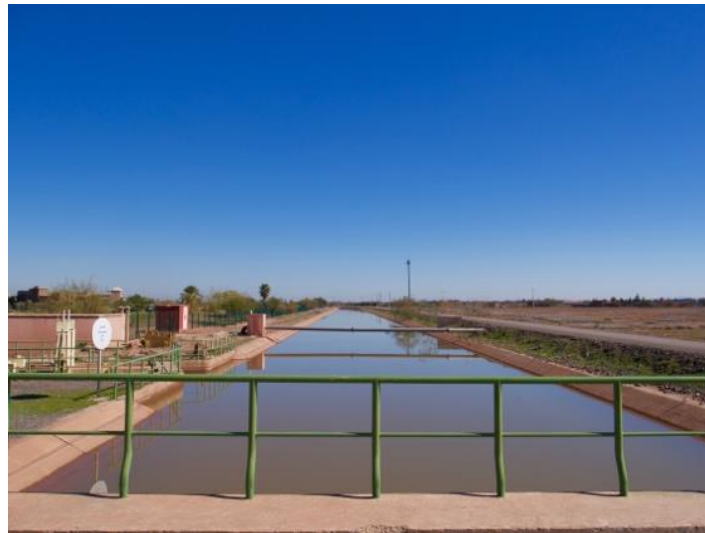
Figure 4-19: Canal System Carrying Drinking Water
