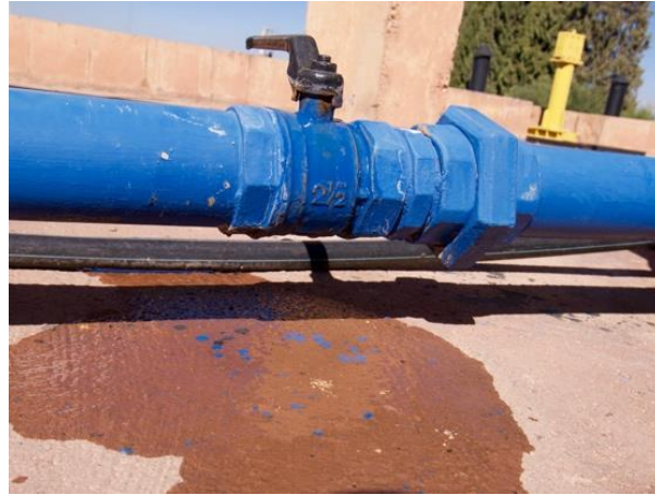
Figure 4-18: Leaking Pipe at Water Filtration Station
