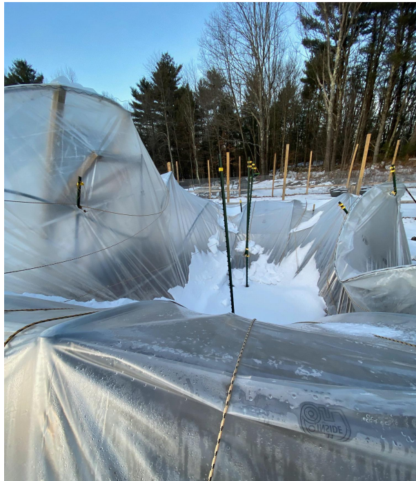
Figure 2: Snow Accumulation and Collapse
