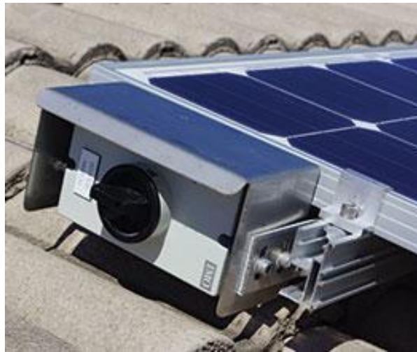
Figure 11: Solar PV System Configuration and Rooftop DC Isolator (Linked Group Services, 2016)
