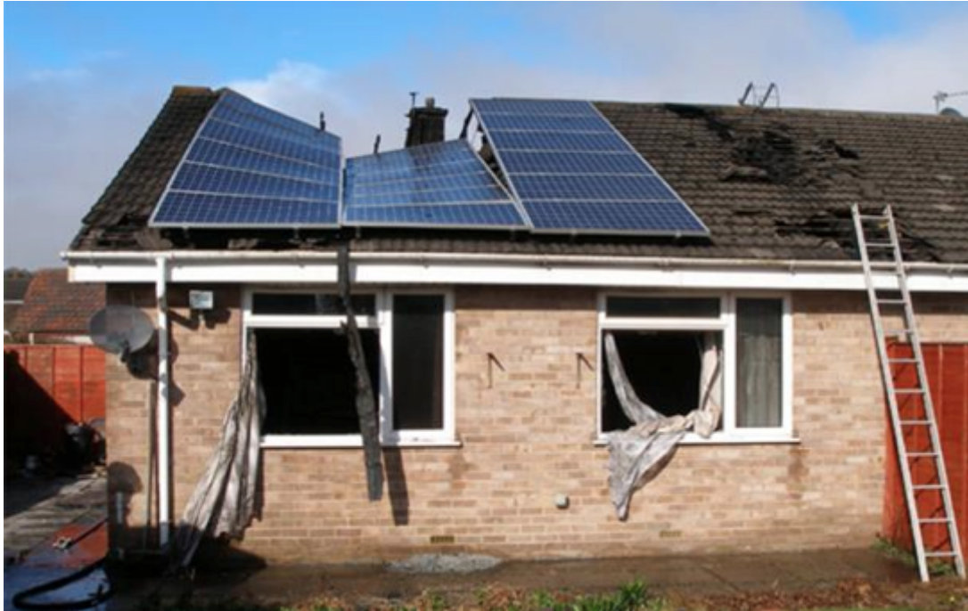
Figure 14: Roof Collapse Cause by Solar PV System Fire (Shipp et al., 2013)
