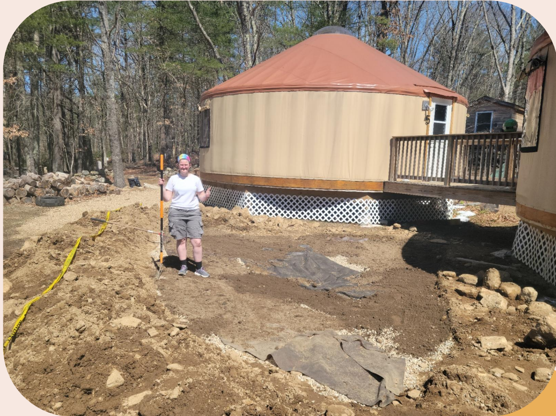
Figure 54: Several rolls of landscaping fabric that were laid down on top of the gravel.
