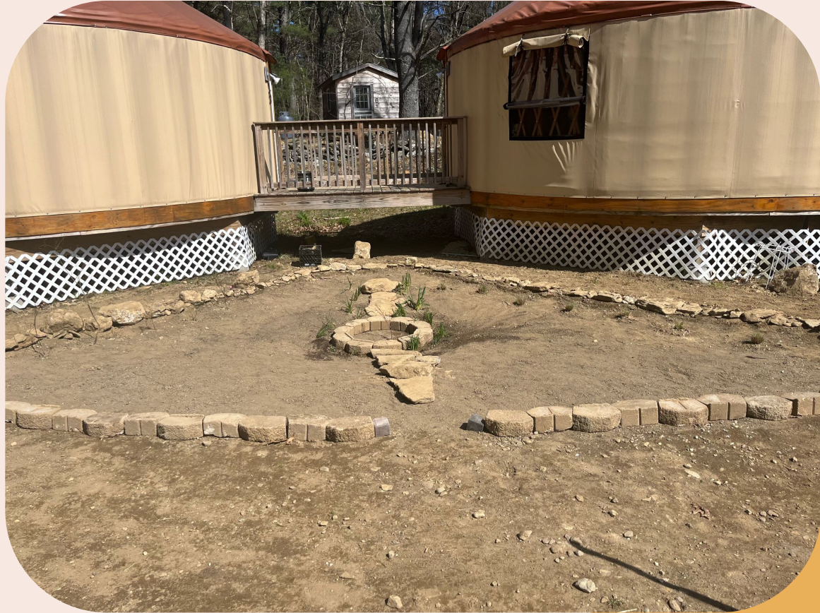
Figure 57: Chives around the red twig dogwood in the center, little bluestems on the right side, highbush blueberries on the left side, and milkweed seeds in the back. Remaining plants hadn't been received yet.
