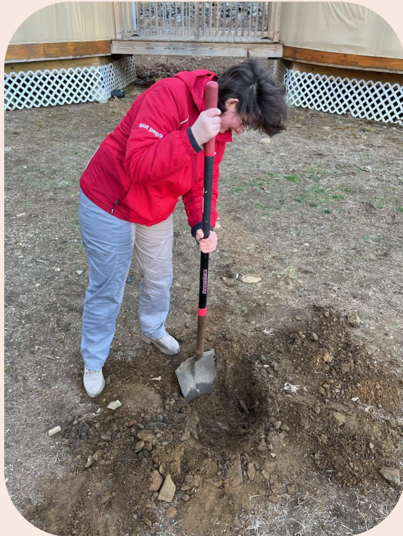
Figure 51: This was taken when we dug two holes in order to test the drainage rate of the site. This determined that we needed to get loam to replace the clay heavy dirt that we dug up later.
