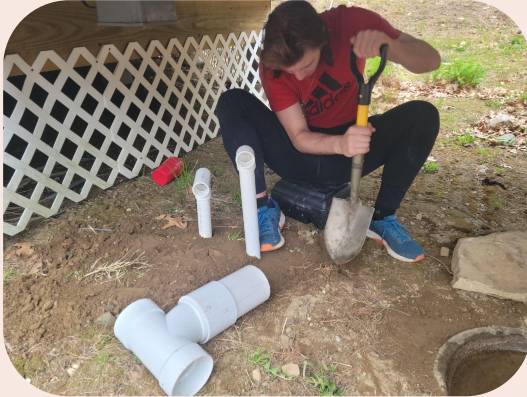
Figure 58: Ethan digging holes for the pipes to go in to create the frog hotel under the bridge.
