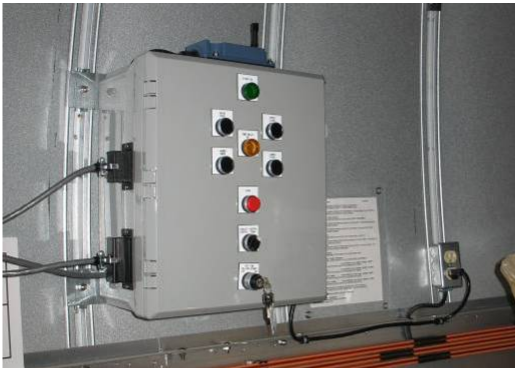
Figure 14: Shutter control panel rides with the dome as it rotates
