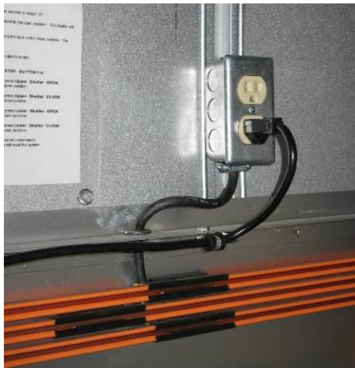
Figure 17: Slip rings move with the dome to power mobile outlet
