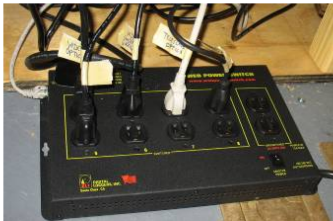
Figure 10: Web Power Switch Installed On-Site
