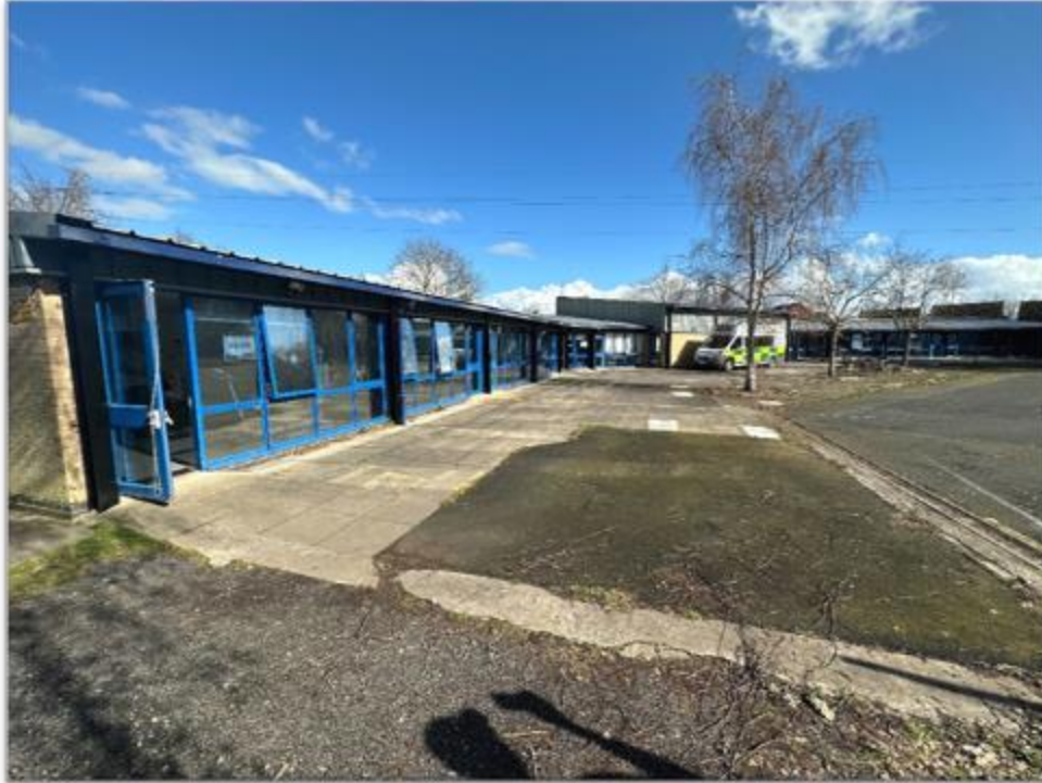
Figure 4.6: A view of the back of the Sheila Scott building. The picture shows many open doors and windows.
