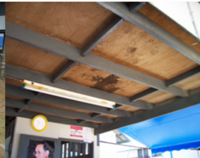
Water marks from rain on the second floor
