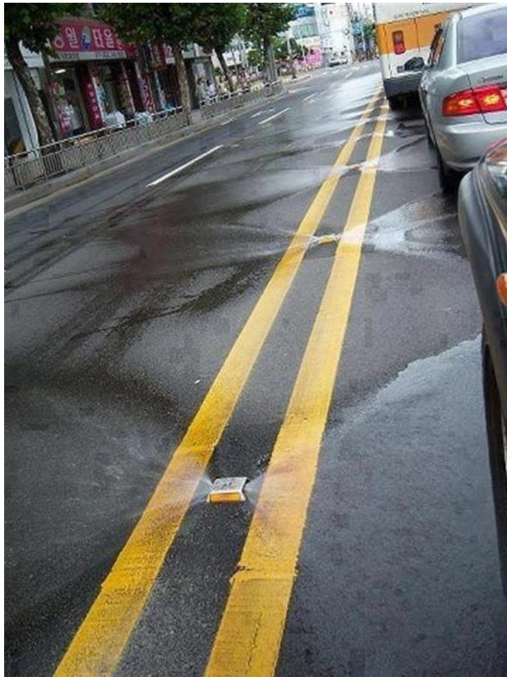
Figure 3 -Road Snow Melting System Tajima
