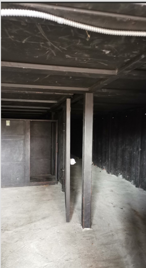
Figure 11: Photo of the labyrinth framework that is in the onsite search and rescue training building.
