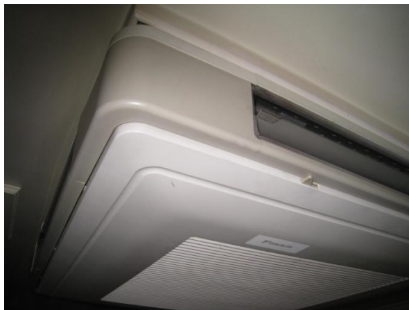
Figure 21 - La Barbe Daikin Air Conditioning Unit
