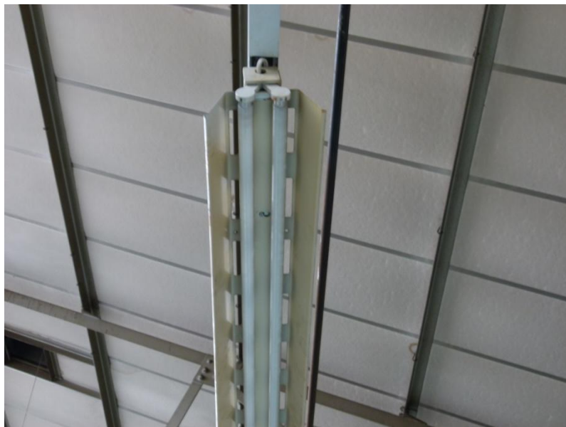
Figure 24 - Risbridger Ltd. Workshop Lighting
