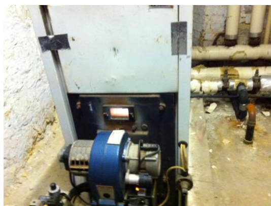
Figure 20 - Wray Park Fire Complex St. David's Gas Boiler
