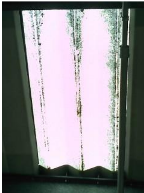
Figure 28 - Armatool Dirty Skylights
