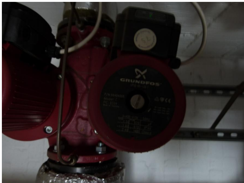
Figure 26 - Risbridger Ltd. Grundfos Pumps
