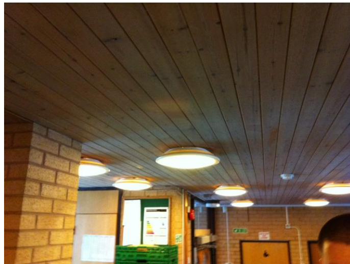
Figure 19 - Wray Park Fire Complex Halogen Lights in Lobby
