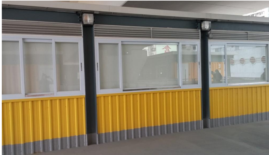
Figure 4.8: Building A - Natural daylight and ventilation not in use
