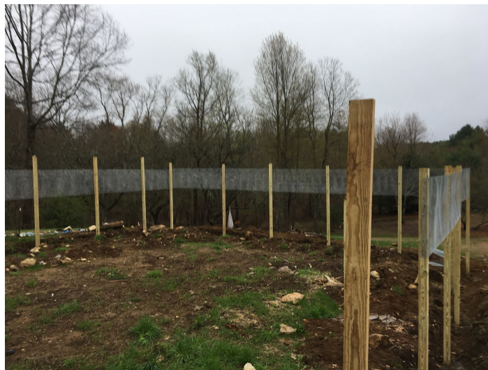
Figure 3e.vii: Fence posts set 2.5 feet in the ground with the top layer of wire mesh netting attached. (Zimak, 2019)
