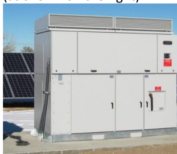
A centralized inverter
