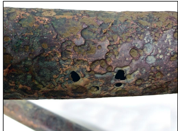
Figure 2. Pitting of a copper pipe (Balkan, n.d.).
