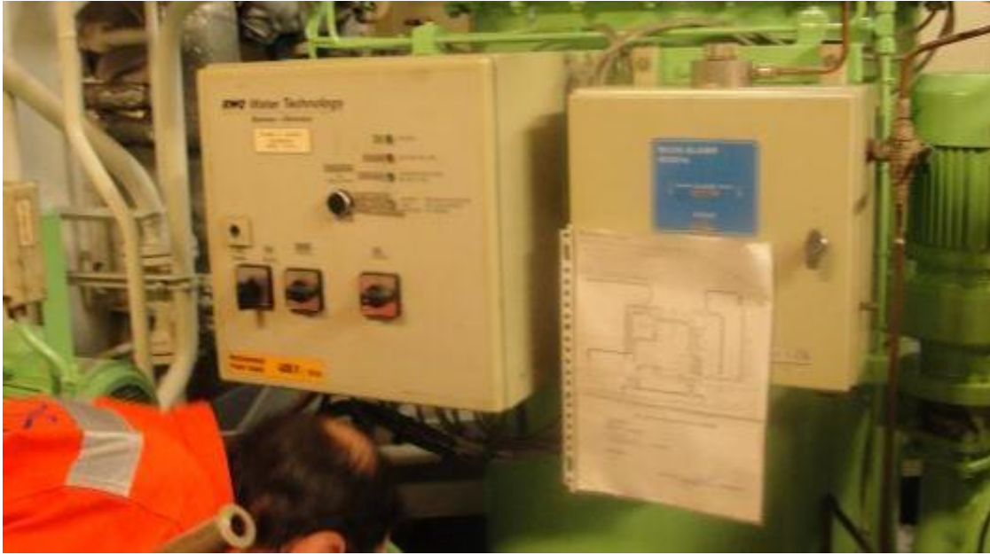
Figure 10: Oil Water Separator
