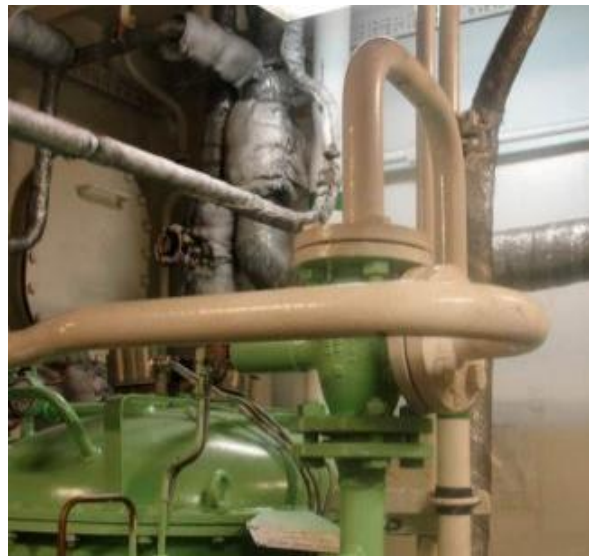
Figure 58: The Valve and Pipe Leaving the OWS.
