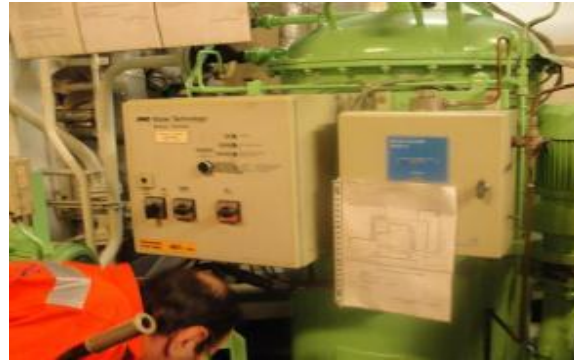
Figure 57: The Oil Water Separator
