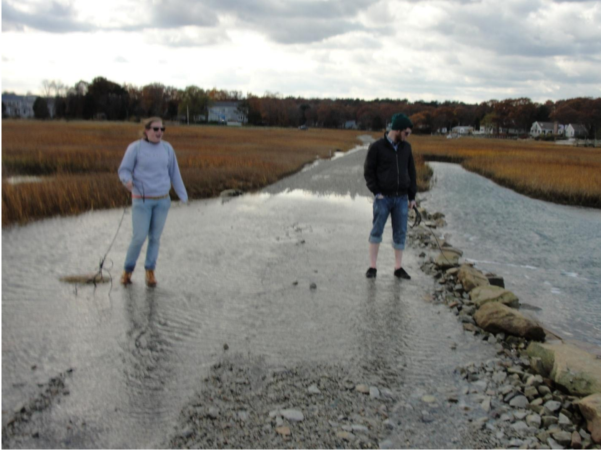
Figure 23: Water flowing over the roadway (Stitt, 2011)
