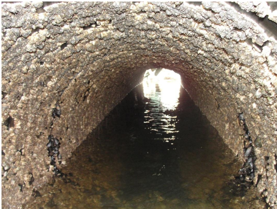
Figure 20: Barnacle cover of Culvert 2 (Stitt, 2011)
