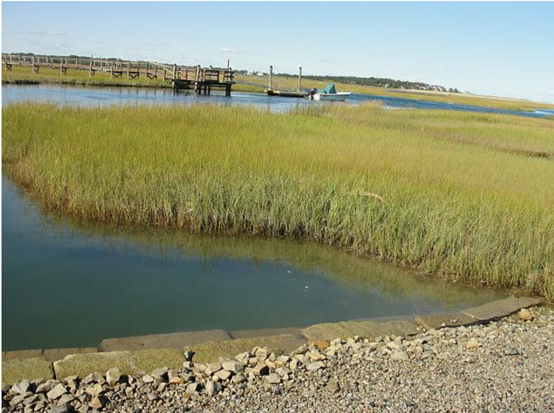
Figure 46. Erosion of the second culvert on the North side of Macomber's Way (Photo source: Brendan Stitt, September 16, 2011)
