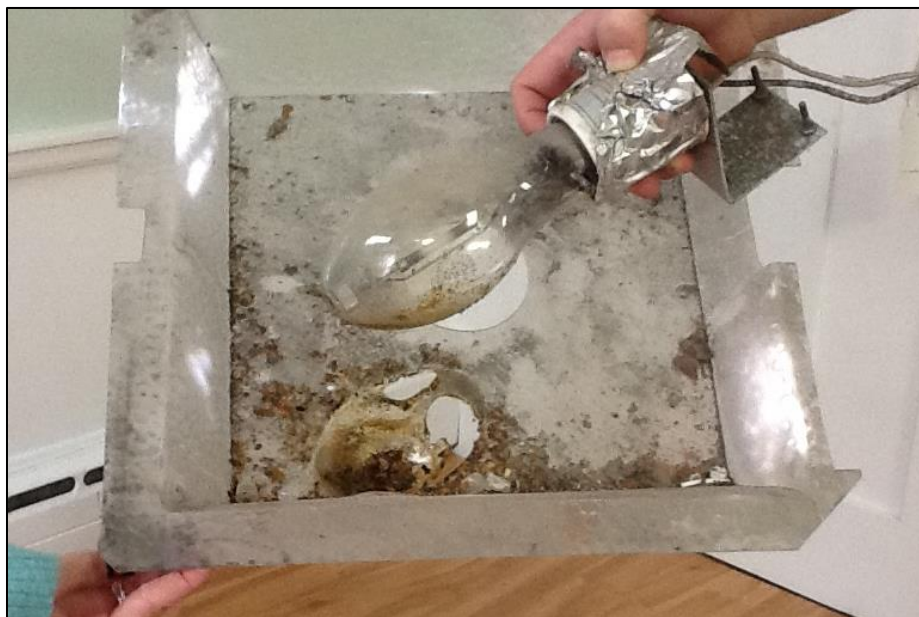
Figure 28 HPS Bulb Melted into Fixture Diffuser
