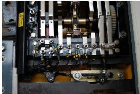
Push rods in point machine
