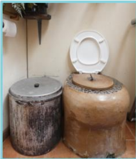
[Picture of a dry composting toilet]
