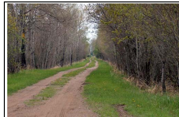
Figure 17: Unpaved Road – Poor Condition
