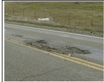
Figure 12: Paved Road - Poor Condition
