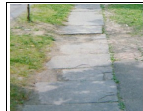
Figure 26: Sidewalk – Below Average Condition
