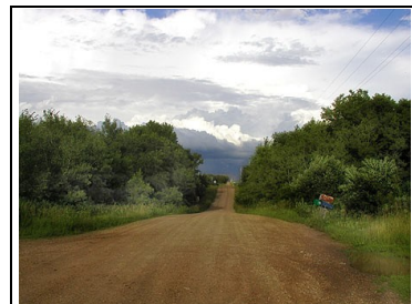
Figure 14: Unpaved Road - Above Average Condition
