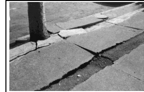
Figure 27: Sidewalk – Poor Condition
