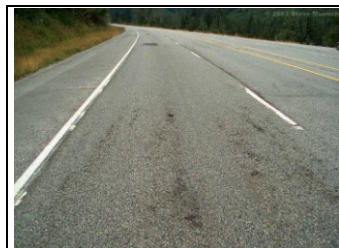
Figure 11: Paved Road - Below Average Condition
