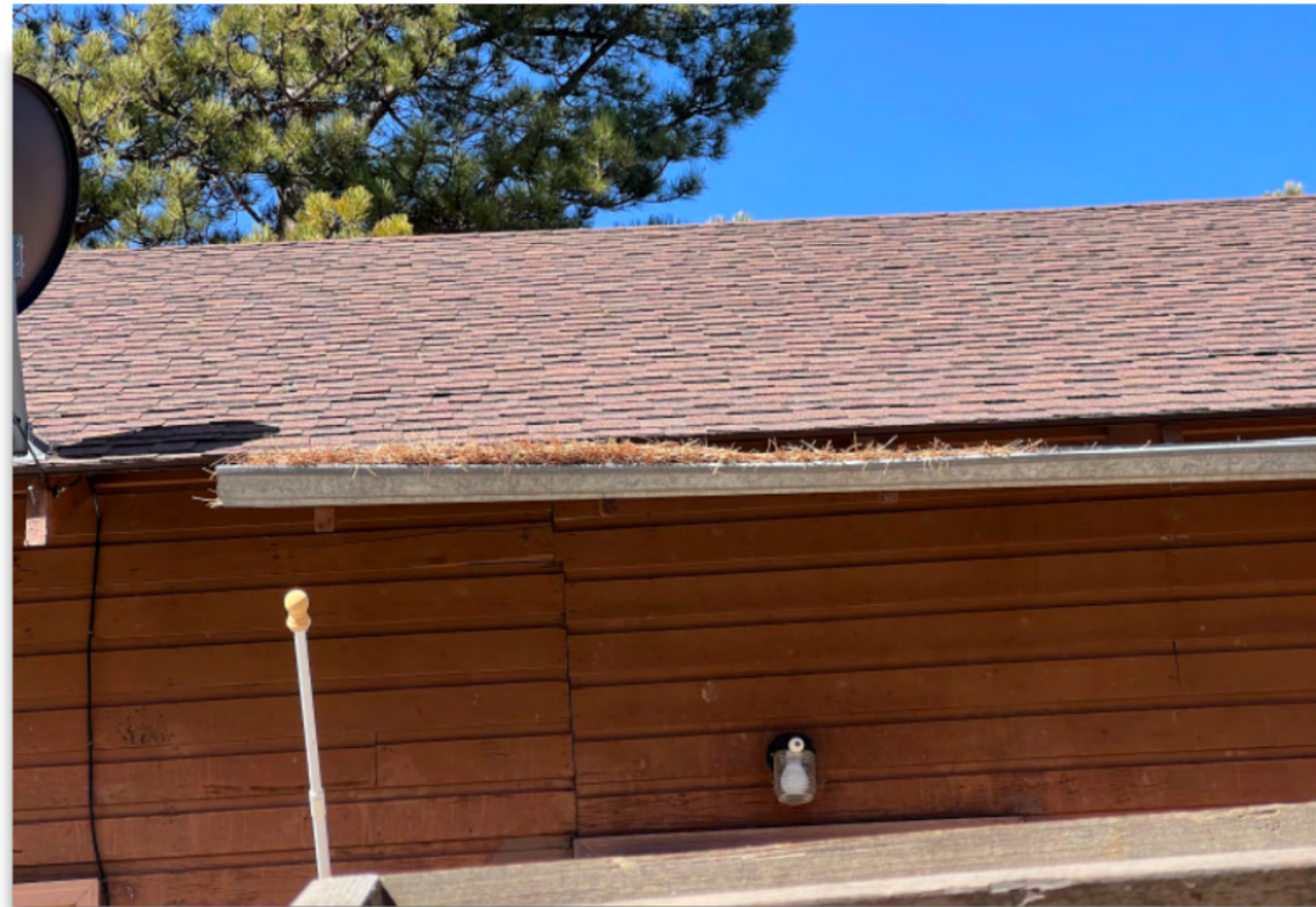
Figure 32: Photograph of cabin with filled gutters
