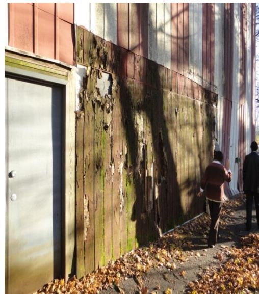
Figure 4: Outer wall conditions of the warehouse
