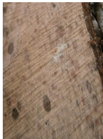
Figure 4.2- 11: Damage of Untreated Plantation Pochote Wood
