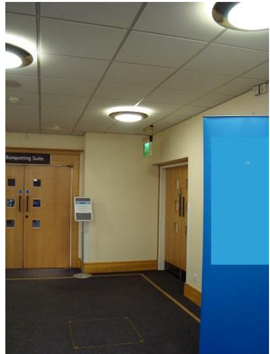
b) Fire exit door in the corridor side, mostly hidden by the blue panel and "competing" with the usual delegate path to go through the double door to a conference room
