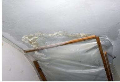
Figure 33: Water damaged ceiling
