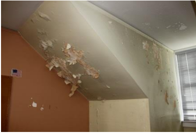
Figure 32: Water damaged ceiling
