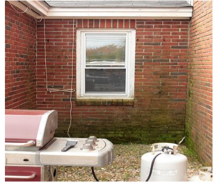
Figure 25: Water damaged brick veneer at main fire station
