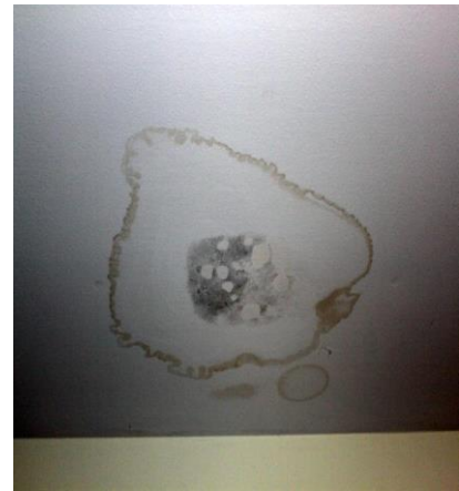
Figure 64: Ceiling leak in the DPW Administration offices
