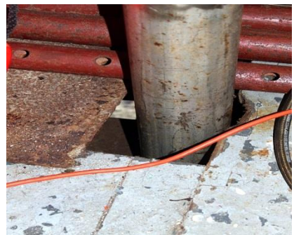
Figure 80: Gap around pillar
