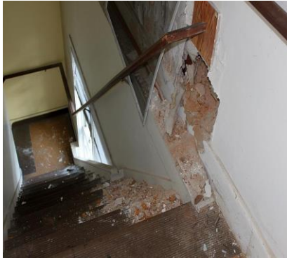
Figure 23: Condemned staircase at 20 South Water St
