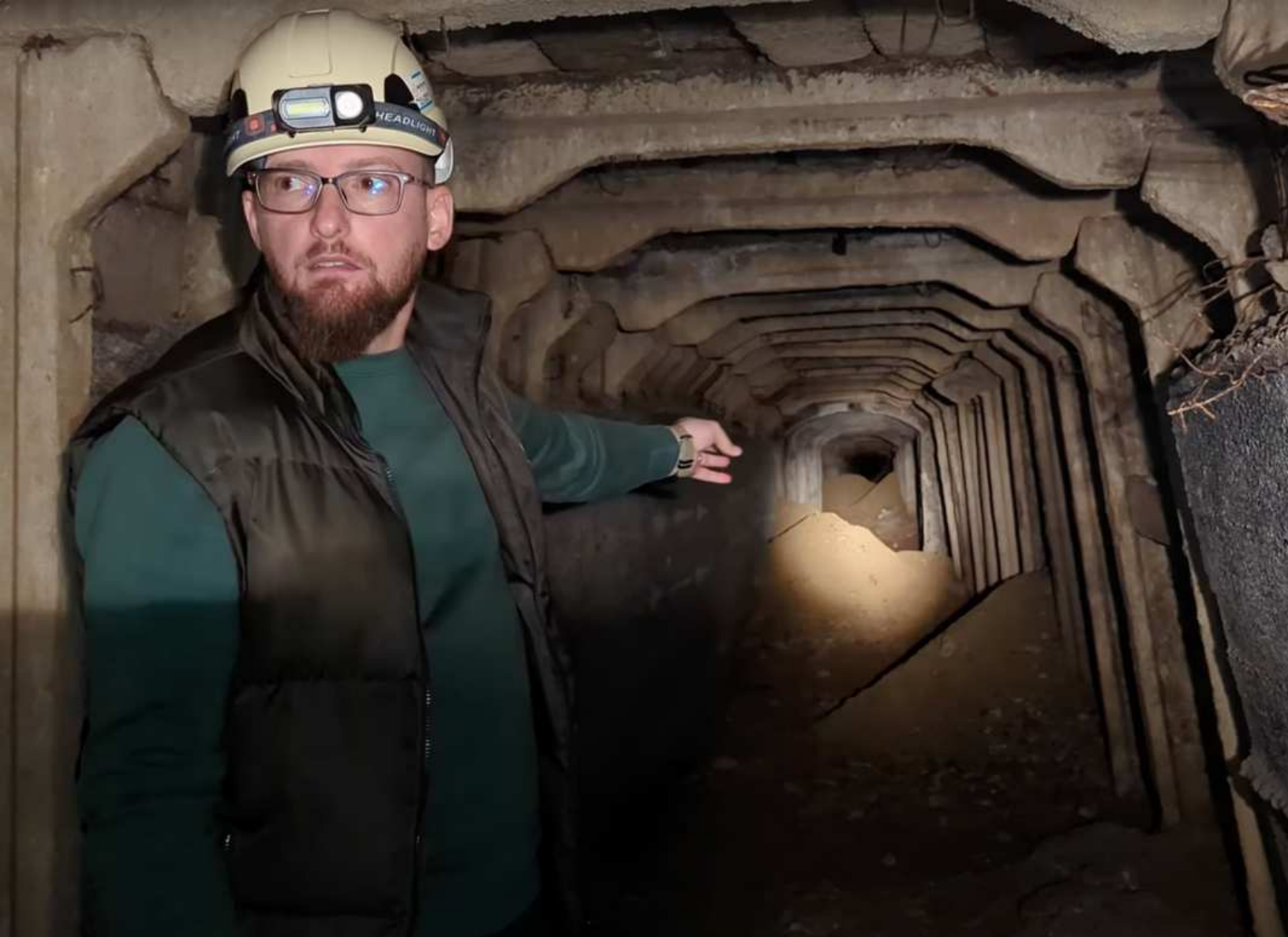
Image 26: Andrit Shehu and the unfinished, deteriorating section of the tunnel network
