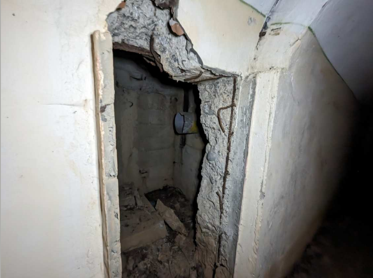
Image 6: Deteriorated section of the underground barracks
