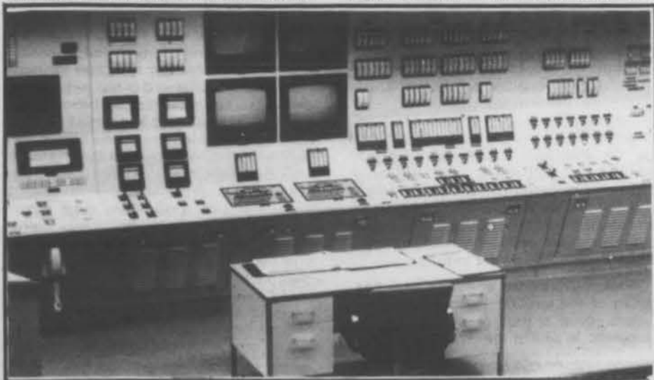
Seabrook's control room.
