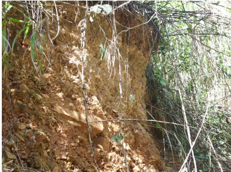
Figure 3: Erosion of the Rio Piedras
