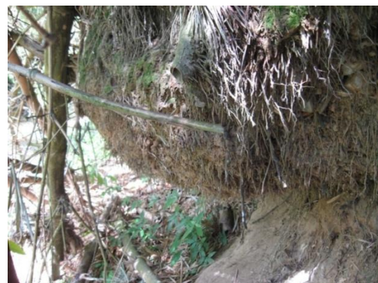
Figure 25: Erosion with Zone 9
