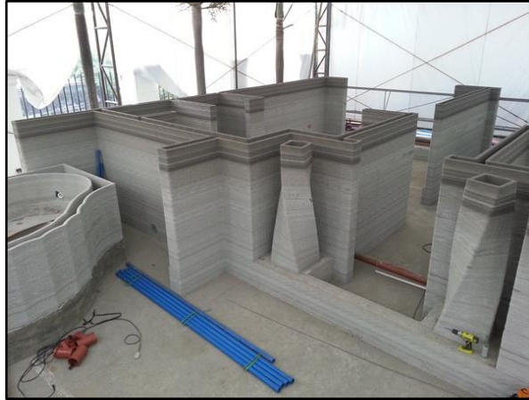
Figure 6: The intricate layout of the 3D printed hotel by Total Kustom (Total Kustom, n.d.).
