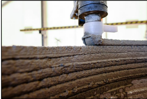
Figure 7: This image is an up-close picture of the COBOD nozzle extruding cement.
