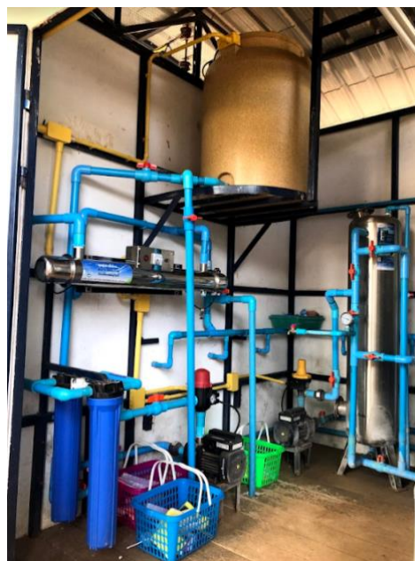
Figure 10. The water filtration systems at Ban Mae Salap including carbon filtration, sand filtration, UF, MF, UV, and RO.
