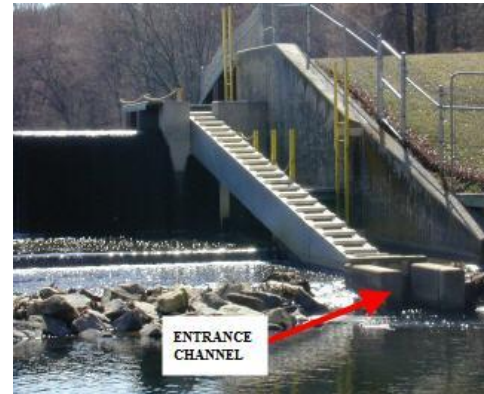
Figure 35. Example Fishway. (Maryland Department of Natural Resources 2007)
