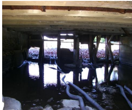
Figure 14. From beneath the bridge and gate house. PVC Pipes and gate house supports.
