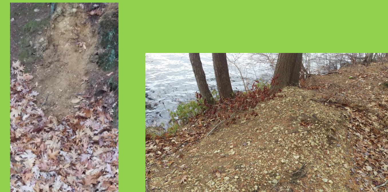
Erosion observed at the Reservation
