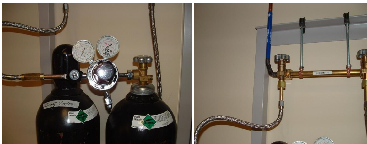
Figure F.4: Nitrogen Supply Valves
