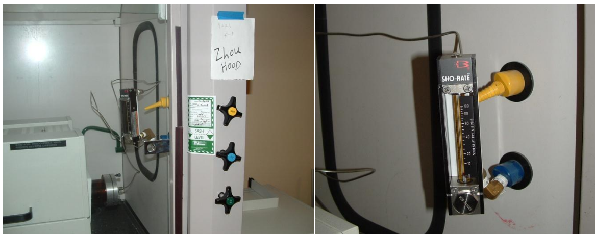
Figure F.5: Nitrogen Control Valve and Flow Meter
