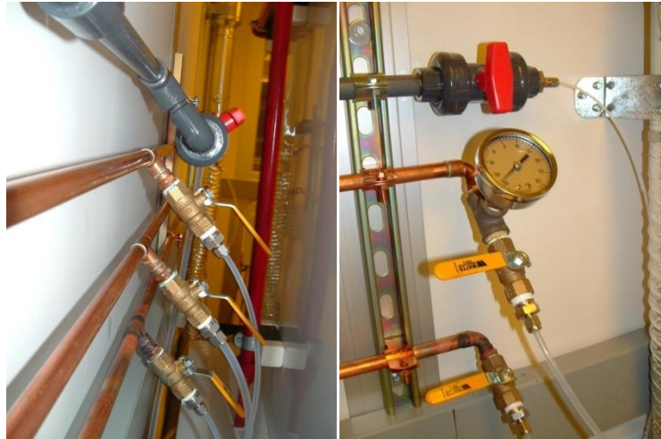
Figure D.4: Hood Supply Lines (Left) and Spin Coater Supply Lines (Right)
