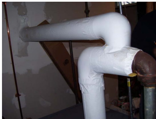
Figure 5: Properly Insulated Piping
