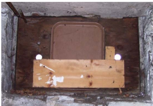
Figure 12: Improperly Sealed Window
