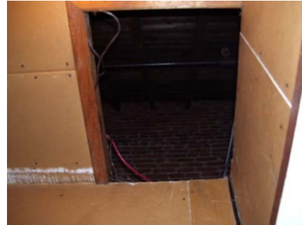
Figure 9: Missing Attic Hatch
