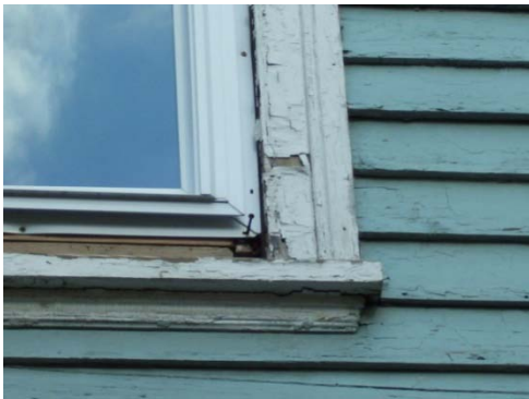
Figure 6: Damaged Window Frame
