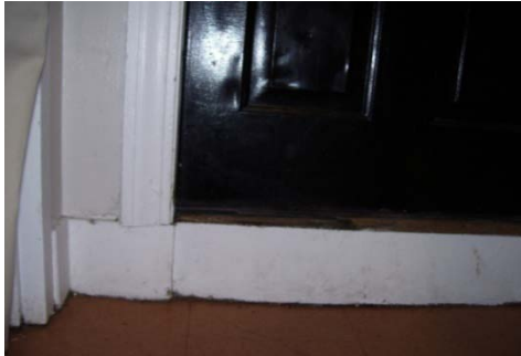
Figure 8: Missing Door Skirt
