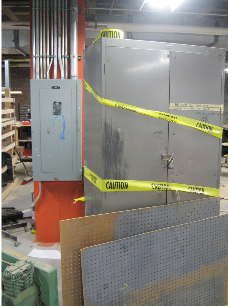
This metal cabinet used to hold all our tools, now they're stored under work benches.
