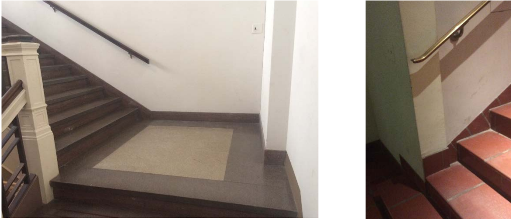
Figure 24: Handrails that are not ADA compliant
