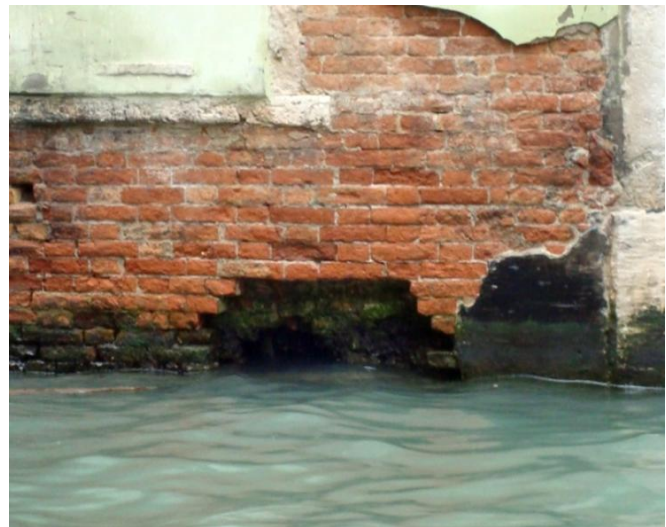
Figure 12: Moto ondosso damage
